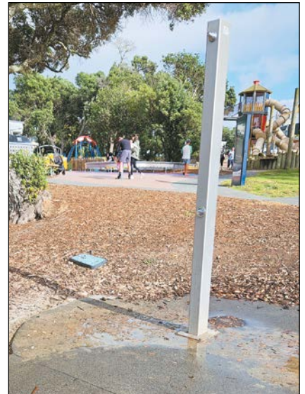
Trickle down... The double-sided shower has a drain on one side, but not the other
